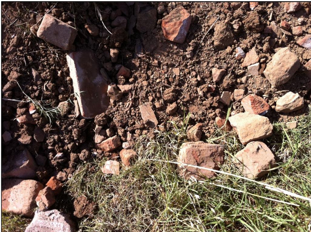
Plate 6 – ACM observed within fill material from Testpit A1.
